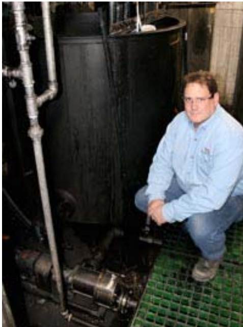
Tim Kreitz, Project Engineer for Rock-Tenn's St. Paul Mill Recycling Center, kneels next to the Blackmer C-Series Eccentric Disc Pump.
