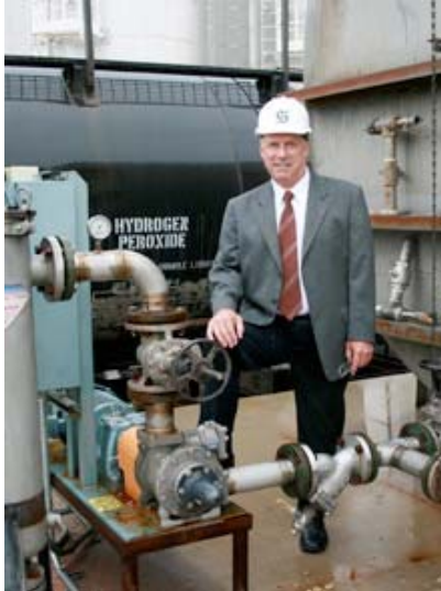
Glenn Gibisch, 3 Rivers' Executive Vice President and COO, stands next to one of several Blackmer pumps at the terminal.
